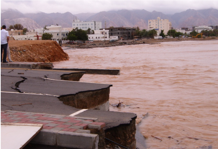
Photo (6) damaged area in Muscat
