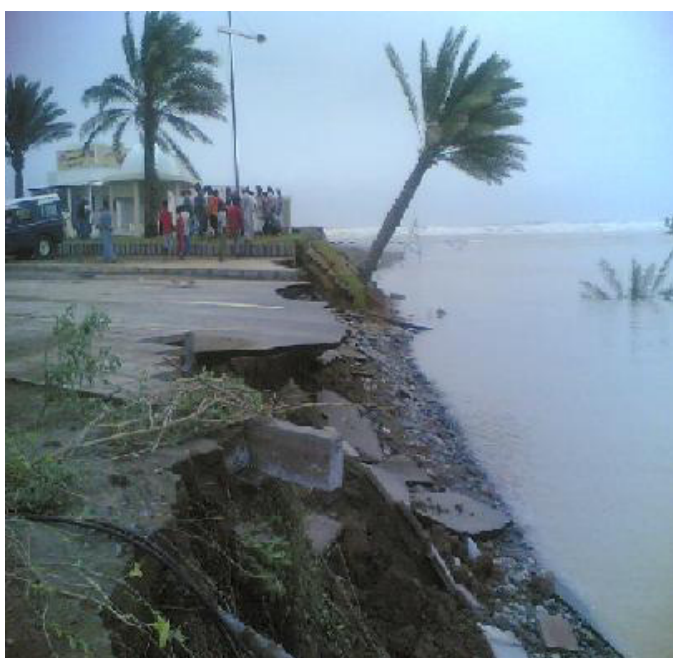
Photo (3) damages on Alqurm beach
