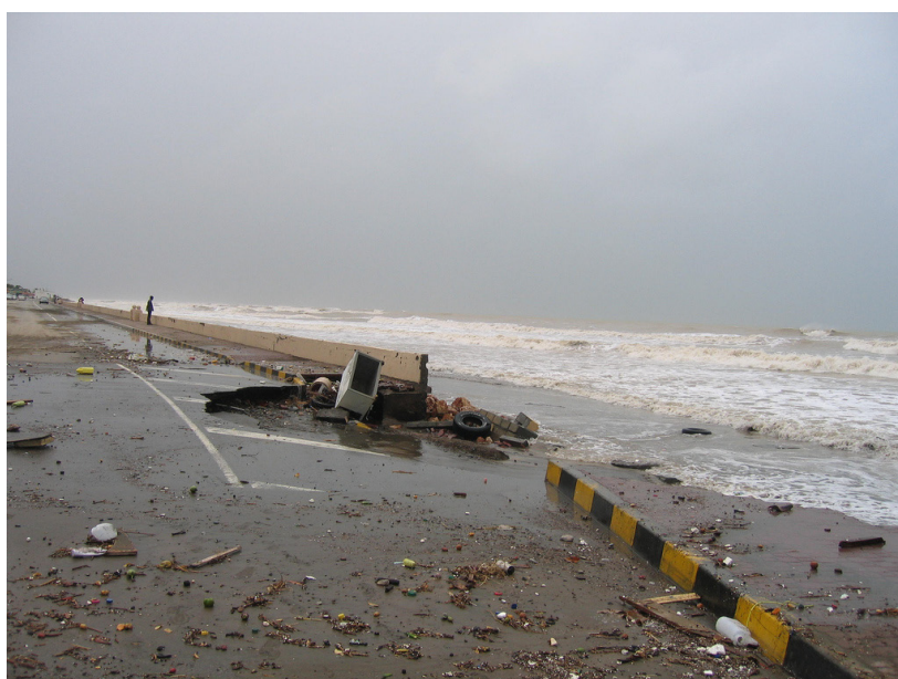
Photo (5) part of damaged beach in Alseeb
