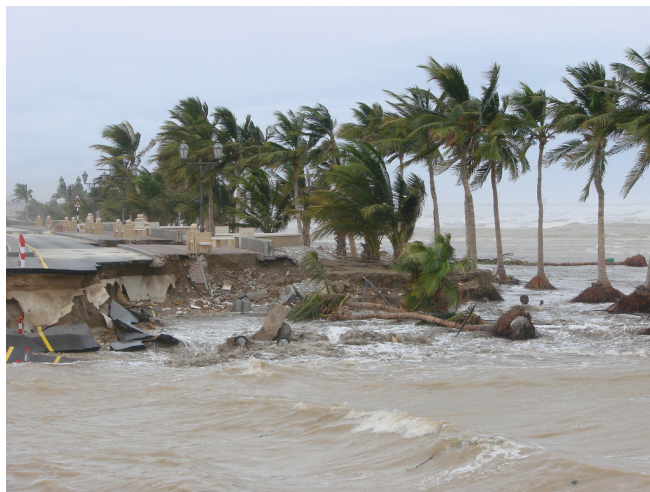
Photo (2) damages on Alqurm beach
