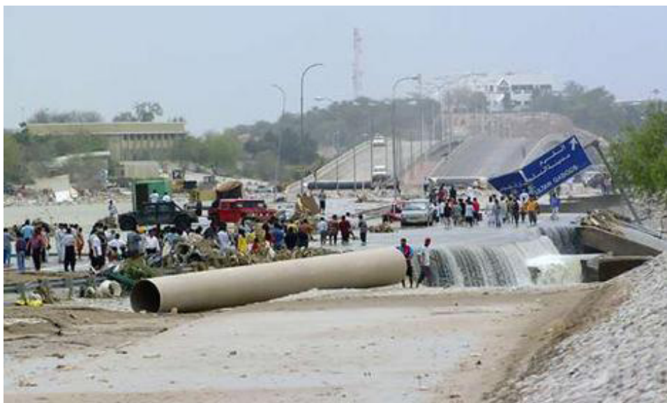
Photo (4) one of the damaged road in Muscat
