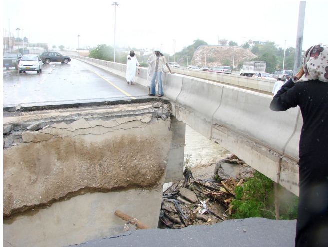
Photo (1) the damaged part of the bridge
